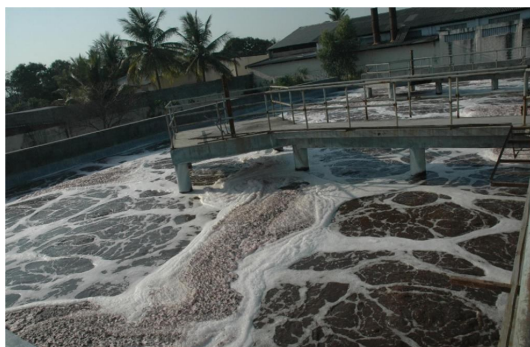
Upgraded aeration tank in SIDCO I CETP
