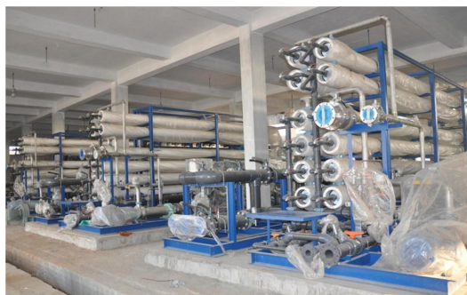
RO installation at Ranitec CETP
